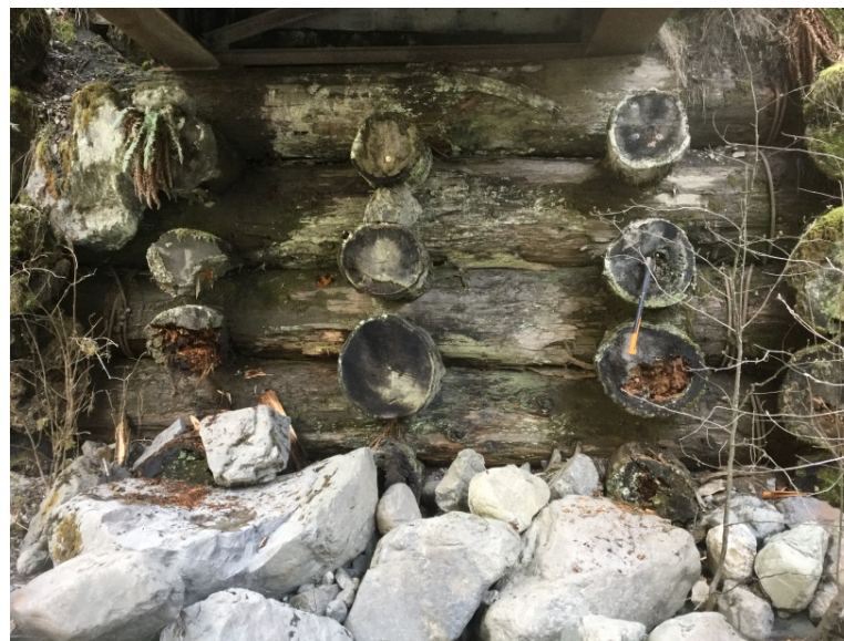
Crib condition at left bank
